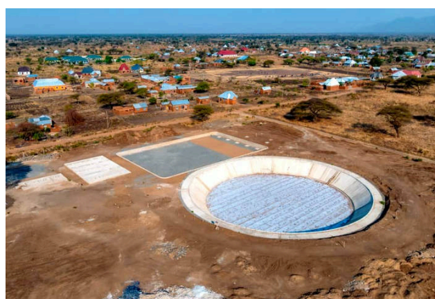
— Sewage system, Mizengo Pinda Campus, Katavi
